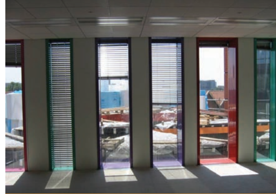
Motorized blinds automatically control incoming daylight.
